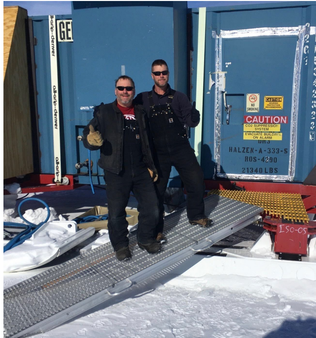
Figure 5. McMurdo team working on generators and power distribution module. The generators and PDM are used to power all the drilling and installation equipment.
