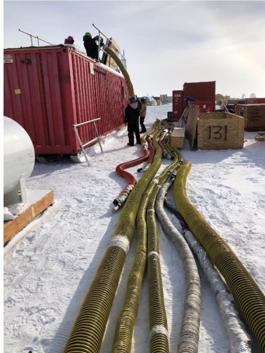
Figure 9. Team laying out heated hoses used to carry unheated water from water tanks to heater modules. Heated hoses ensure against water freezing between the modules.
