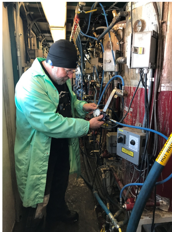
Figure 6. James Roth testing main heater control system elements. The main heaters are used to increase the water temperature to near boiling point before it is delivered to the hose reel and drillhead.
