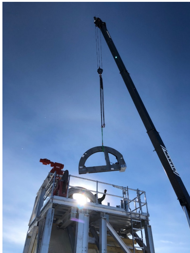
Figure 8. Graham Roberts marshalling during hose crescent installation. The hose crescent guides the main hose over the drill tower as it points downward into the hole.
